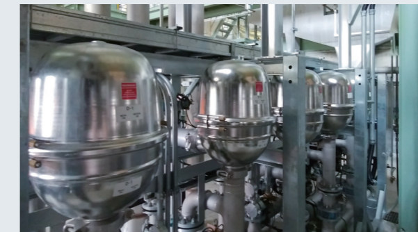
Filtration device installed at the Niigata Mill
