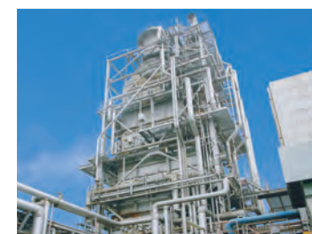
Kanto Mill (Ichikawa) Gas heat exhaust boiler
