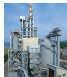
Kishu Mill Wood biomass boiler
