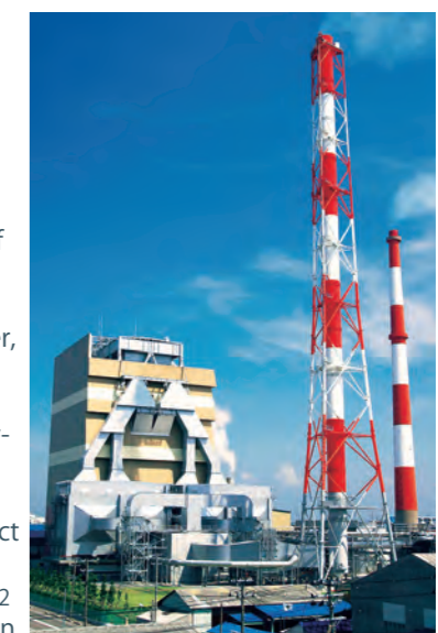
No. 8 recovery boiler at the Niigata Mill
