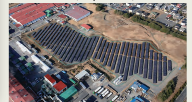
Solar power generation facility at Kanto Mill (Katsuta)
