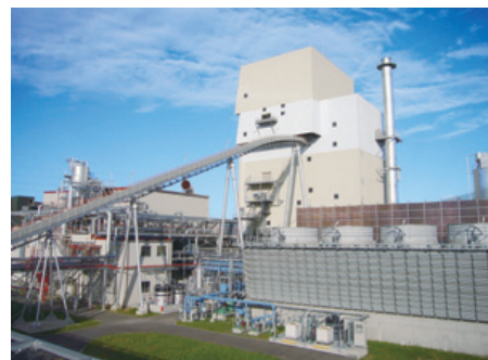
Japan's largest biomass boiler at the Kanto Mill Katsuta
