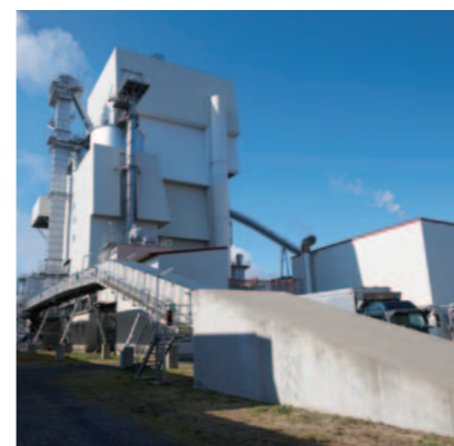
A biomass boiler in the Kanto Mill Katsuta with the power generation capacity of 41,000kW. It generates more than twice as much electricity as is needed by the Mill during peak-time usage, so the excess power is sold externally.
