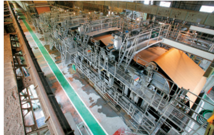
No. 5 papermaking machine at Kanto Mill Ichikawa
