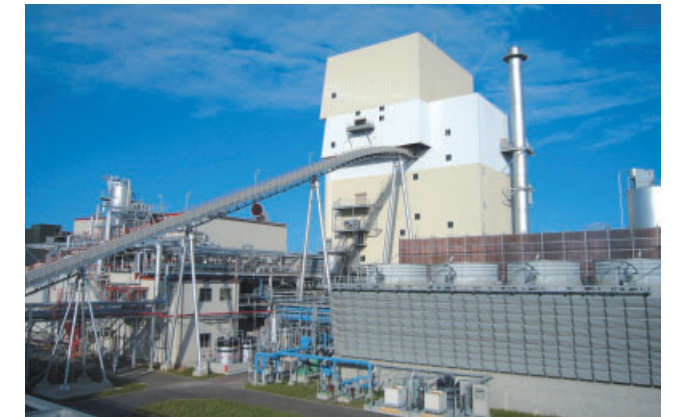
勝田バイオマスボイラー／Biomass boilers power generation plant at Katsuta Factory
