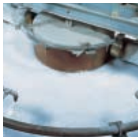
古紙の高度処理設備 Advanced facilities for processing used paper
